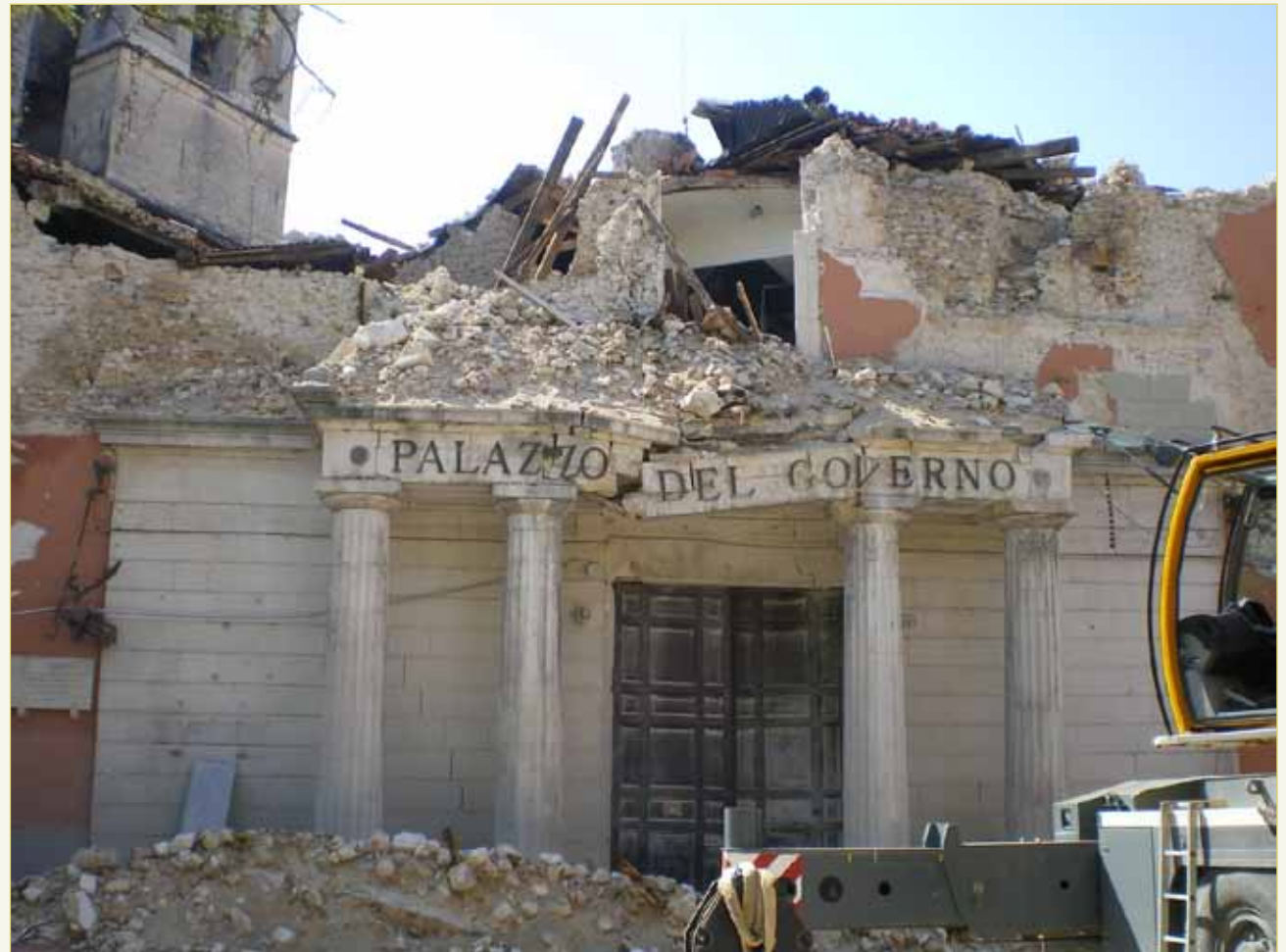
The local prefecture, a government office, damaged by earthquake.
